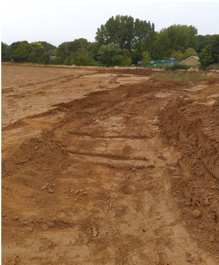
Photograph shows an excavation by a landowner to form a ditch adjacent to the community centre.
